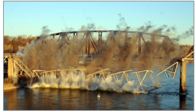
Demolition of the first section of the old Rulo bridge. Photo by Jason Schock
